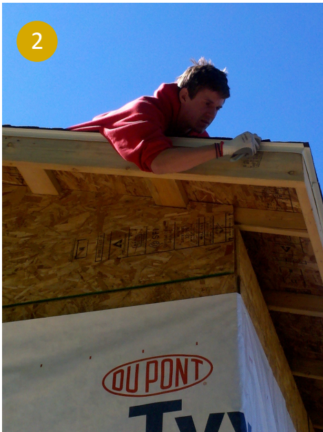
Austin B. is stripping the asphalt shingles to align evenly with the edges of the roof.
